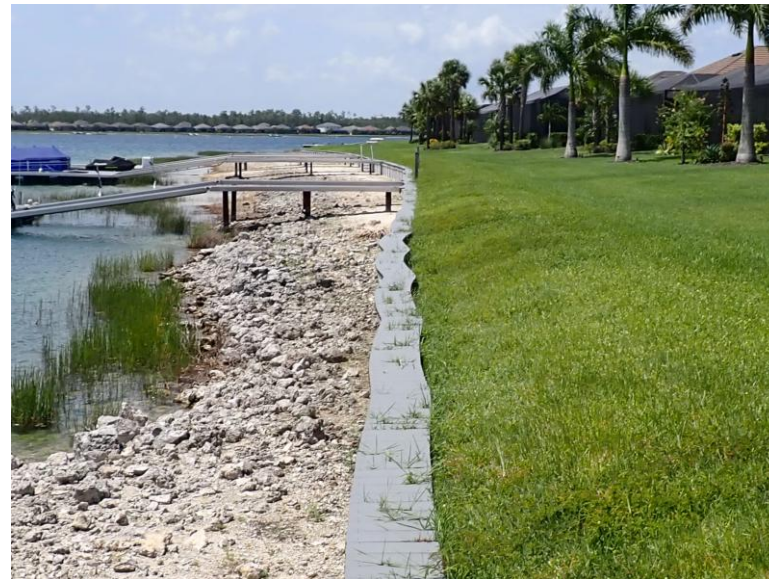
Retaining wall “intact but undulated”
