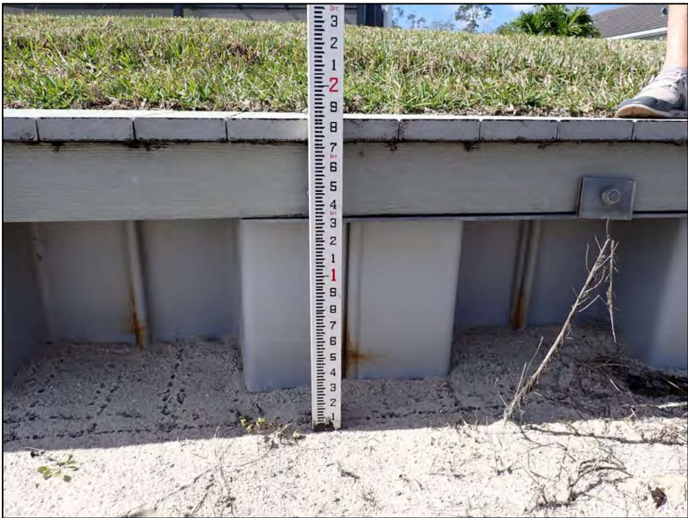
Photo 3. Seawall exposed height of approximately 1.85 feet.
