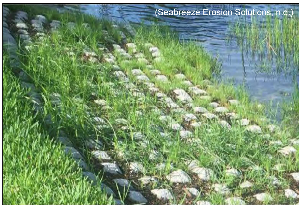
Photo 10. Vegetation growing through a concrete erosion control mat.
