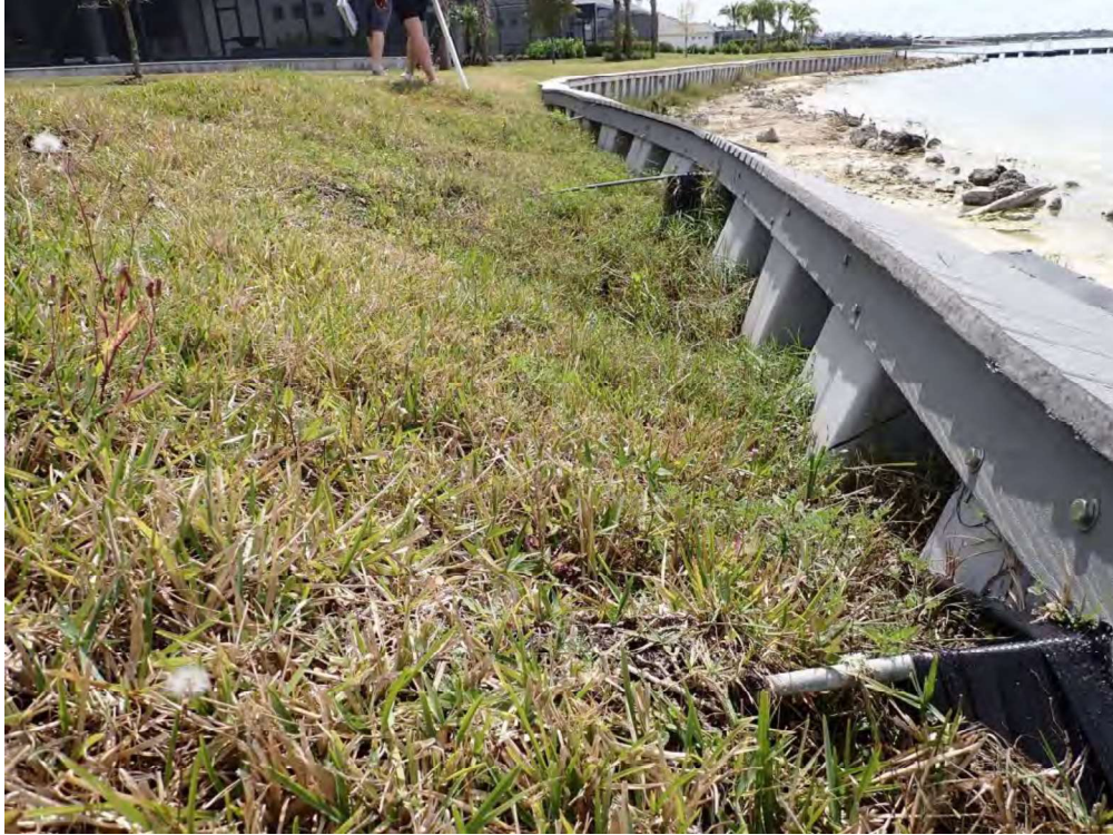
Photo 5. Severe waterward rotation and wall failure.
