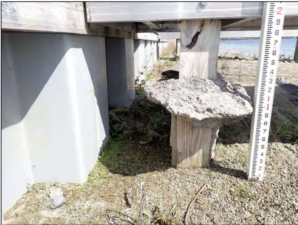
Photo 6. Sediment erosion on a dock piling.
